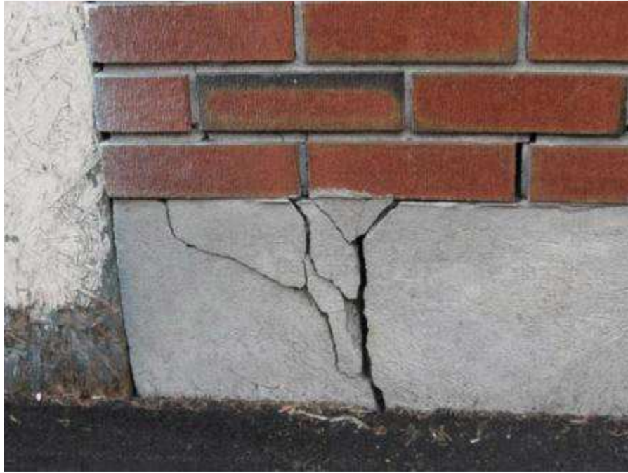
Damage from swelling clays can range from stuck doors and windows to severely buckled walls, floors, foundations, roadways, and commercial structures.
