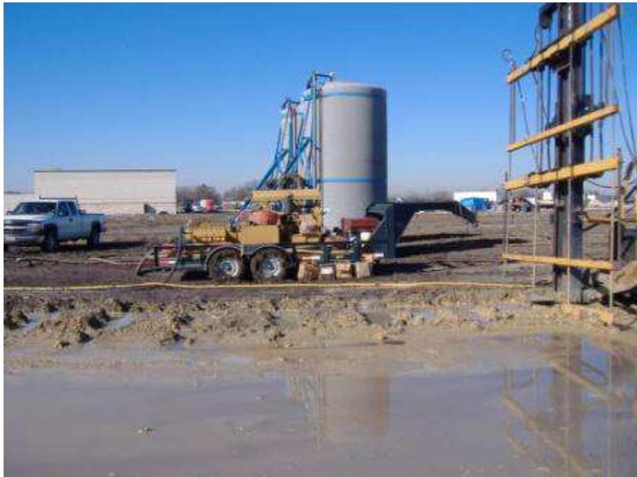
Pre-treating an entire project site with an electromechanical stabilizer can allow a development to function as though clay soils were non-existent.
